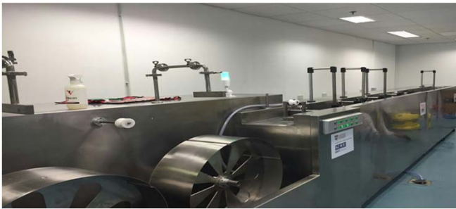
Commercial level hollow fiber spinning line
