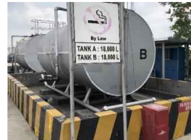
Land based fuel storage tank
