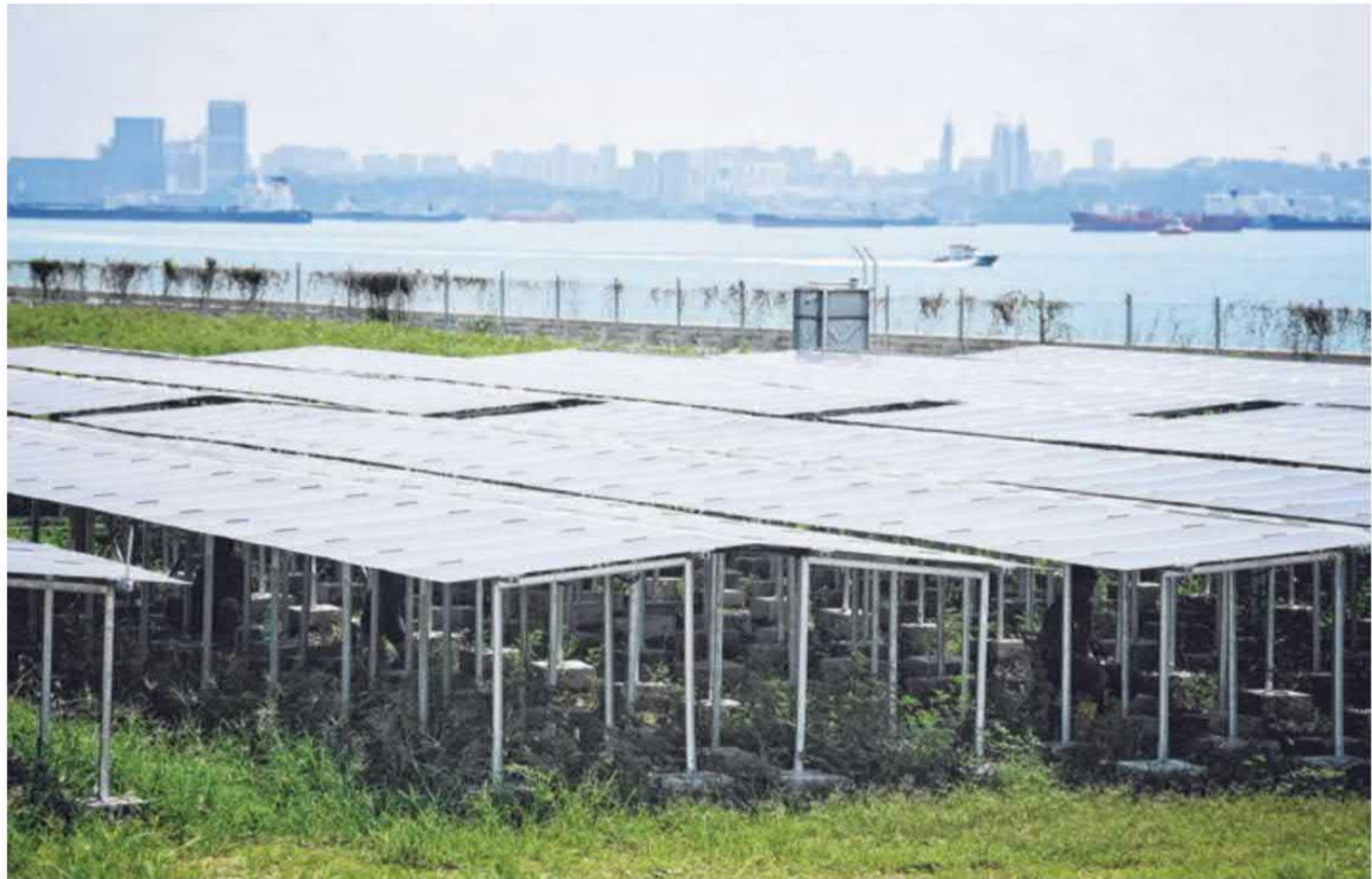
Solar panels at Nanyang Technological University's Renewable Energy Integration Demonstrator-Singapore site on Semakau Island. The micro-grid system, the first of its kind in South-east Asia, serves as a platform for companies to test research projects that are powered by renewable sources of energy in real-world conditions. ST PHOTO: MARK CHEONG
