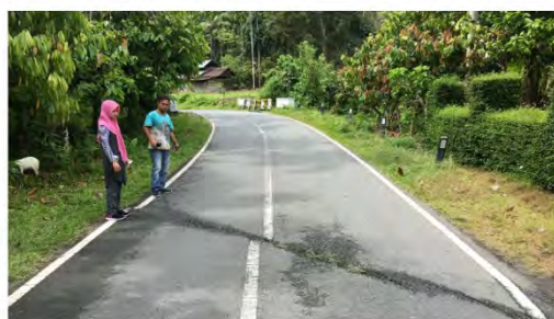
The surface trace of the Sumatran fault cuts across the road between the communities of Mane and Tampo in Aceh, Indonesia. Credit: Qibin Shi
