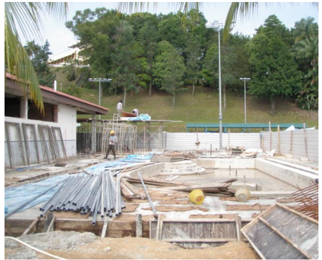
Wading Pool as on 02.11.09 (with laying works being carried out around the pool)
